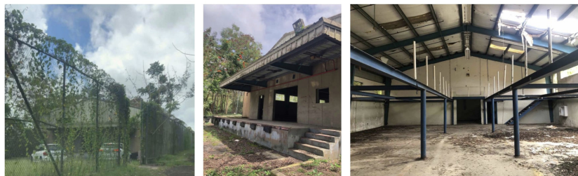
Fig. 2. Existing Conditions of Abandoned Structure (Perez and Vargas, 2021)
