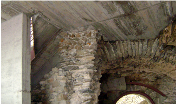
Fig. 3. Contemporary intervention without dialogue with the preexisting structure. Insertion of a new reinforced concrete slab and “pilotis” (columns) into a space originally conceived as vaulted. Excessive discernibility (material and formal), even in the reinstatement of the arches (photograph by the author).
