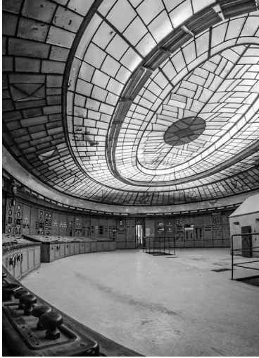
Fig. 2. Control room of the Kelenföld power plant, Budapest, Kálmán Reichl with Virgil Borbíró (photo by the author)
