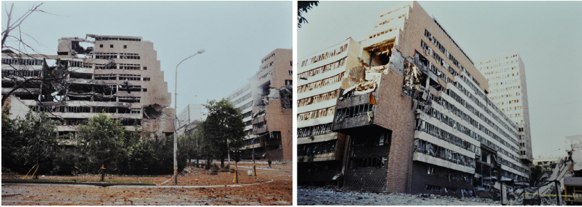
Fig. 2. Damage to the General Staff building immediately after the second bombing (Dragiša Poznanović, 1999)
